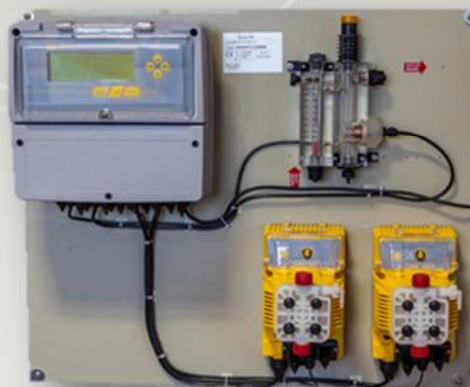
Helios 05 with 2 pumps
